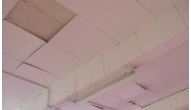
Conference room: Ceiling tiles slowly coming off
